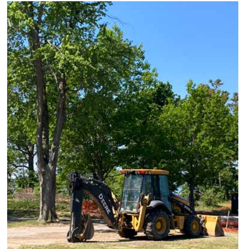
This tree is not adequately protected from ongoing construction. Heavy machinery driving over roots and parked near trees can compact the soil, damage roots and lead to the decline in tree health or mortality.
