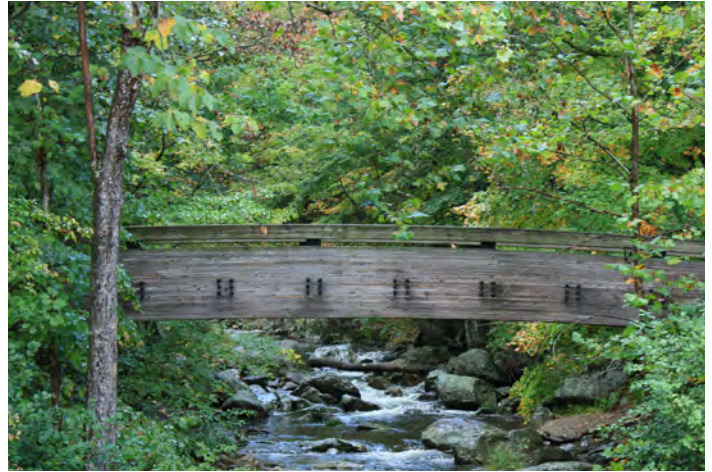
This bridge forms part of a Nelson County, VA greenway trail which provides relaxation and fitness opportunities for nearby residents.
