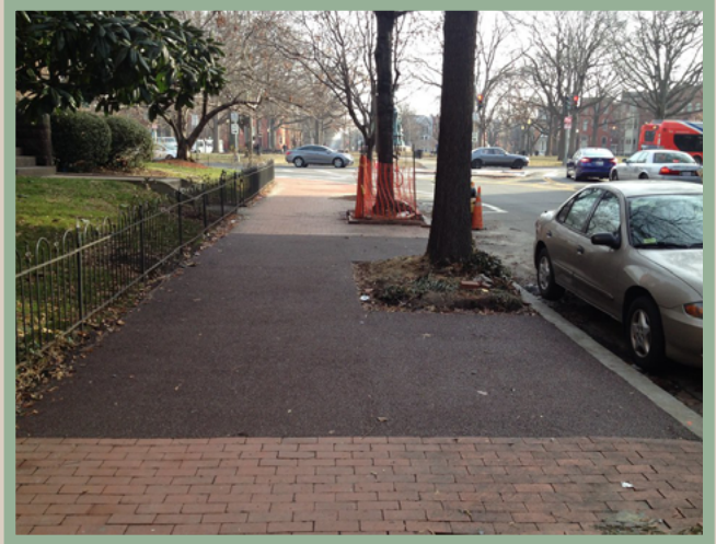
Modifying the sidewalk with alternative permeable or flexible pavement material around the critical roots.
