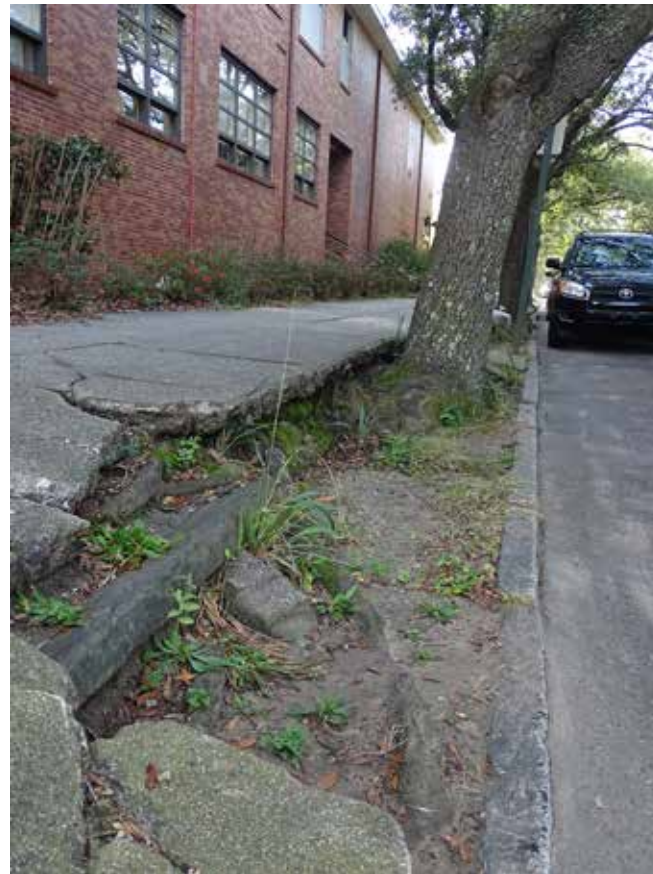
This tree is too large for its planting space and is now causing safety concerns for pedestrians.
