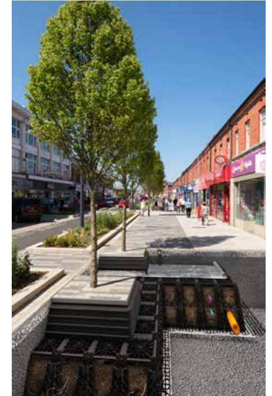
Trees in shopping areas that are heavily trafficked can still be healthy by adding in underground structural supports.
