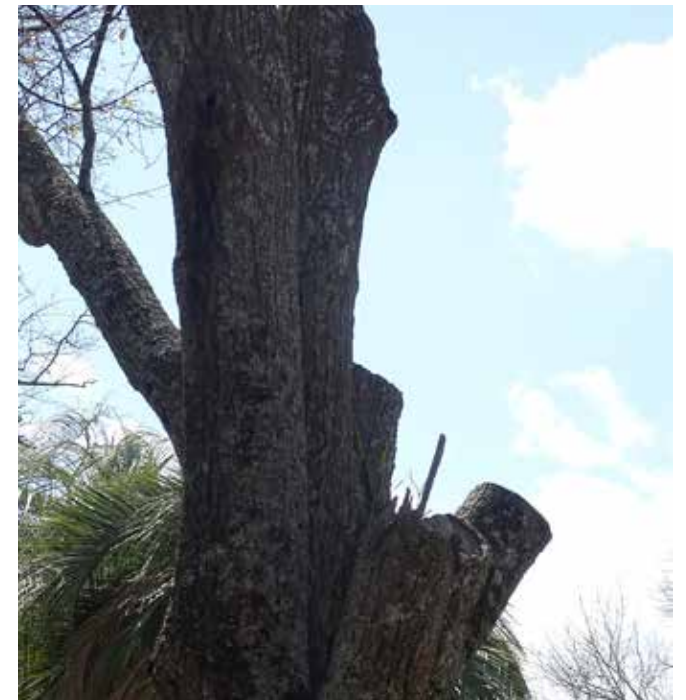
This tree has lost limbs due to storms and is now dead and requires removal to protect public safety.
