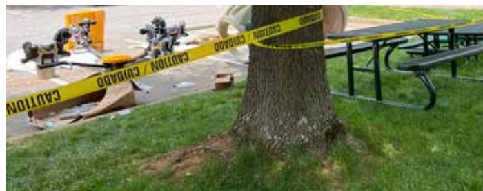
Trees that are not properly protected during land disturbing projects are more likely to experience damage from construction equipment that may lead to decline and death.
