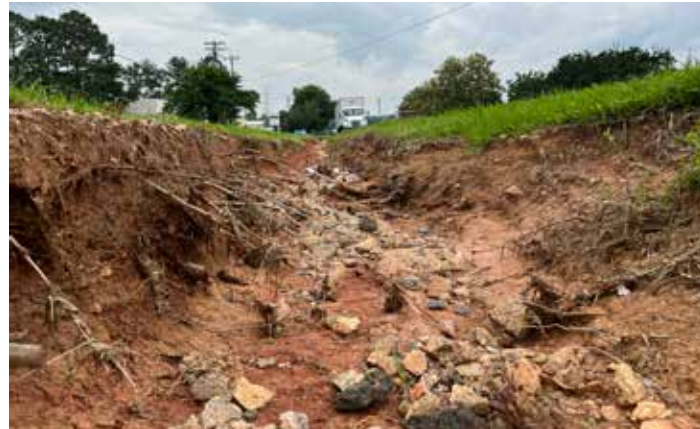
This road shoulder is significantly eroding from surface runoff. Trees help stabilize the soil and prevent erosion.
