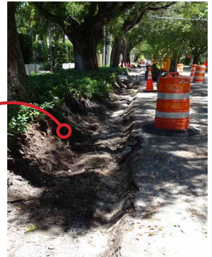
Without using caution, utility work can damage tree roots.
